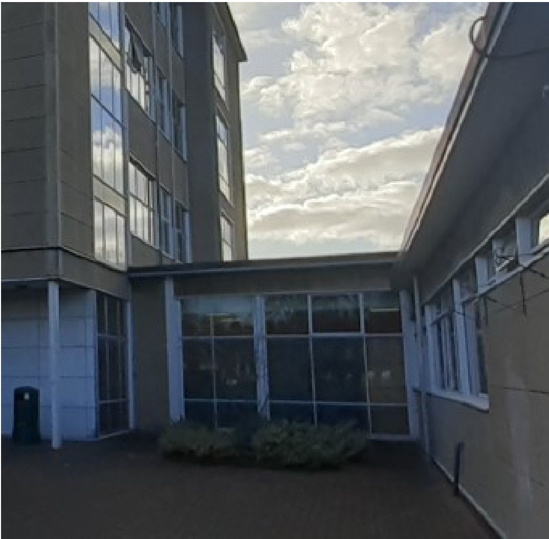
Original metal framed glazed screen details to north elevation of dining space. Image also shows the screen in context to the adjacent screen detail at the base of the stairs. And in the image below the original window details of the catering space
